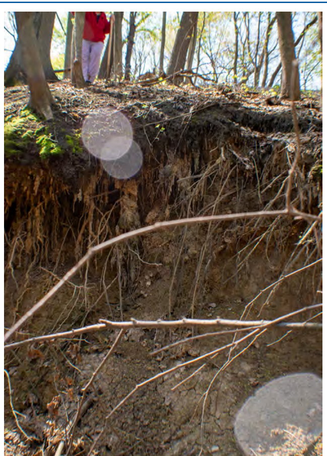
Incised channel below an outdated and poorly maintained stormwater outfall. Such neglect of stormwater infrastructure can cause significant erosion, which contributes to downstream sediment pollution, East Moline, Illinois. Photo credit: Olivia Dorothy
